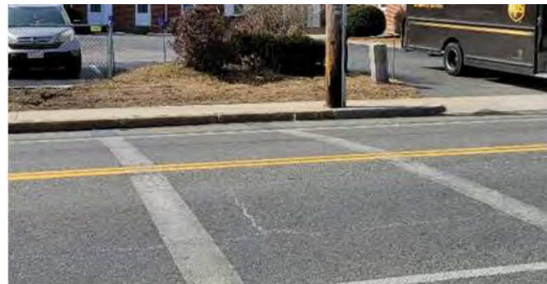
This crosswalk does not lead to a ramp, creating a hazard for those in wheelchairs or with mobility issues.
